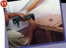
11 While you've still got easy access to the innards of the assembly, fit the shelves...
