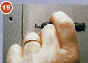
19 Punch the nails well in, leaving plenty of room for the filler to take. The nails are only holding the boards in place while the glue goes off
