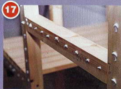
17 Fixing the plasterboard with too many nails means a lot of filling; try using one of the compound glues in a tube in a mastic gun instead
