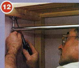
12 ...and hangers. These jobs are much harder once the plasterboard is in
