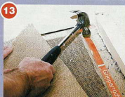
13 Cut your carpet to shape before continuing; here, the gripper rod is going down
