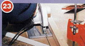
23 Follow the manufacturer's instructions when cutting the worktop; this will probably mean working from the underside. Use a strong, straight board as a guide if you are using a portable circular saw. Cut the mitres first then trim to length, just in case you get it wrong!
